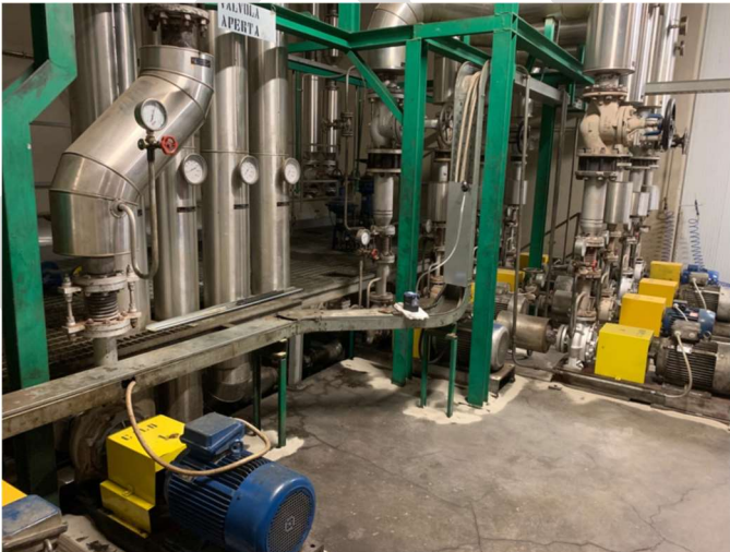
Figure 13. Air sample point in Site S-11 (pumps)
